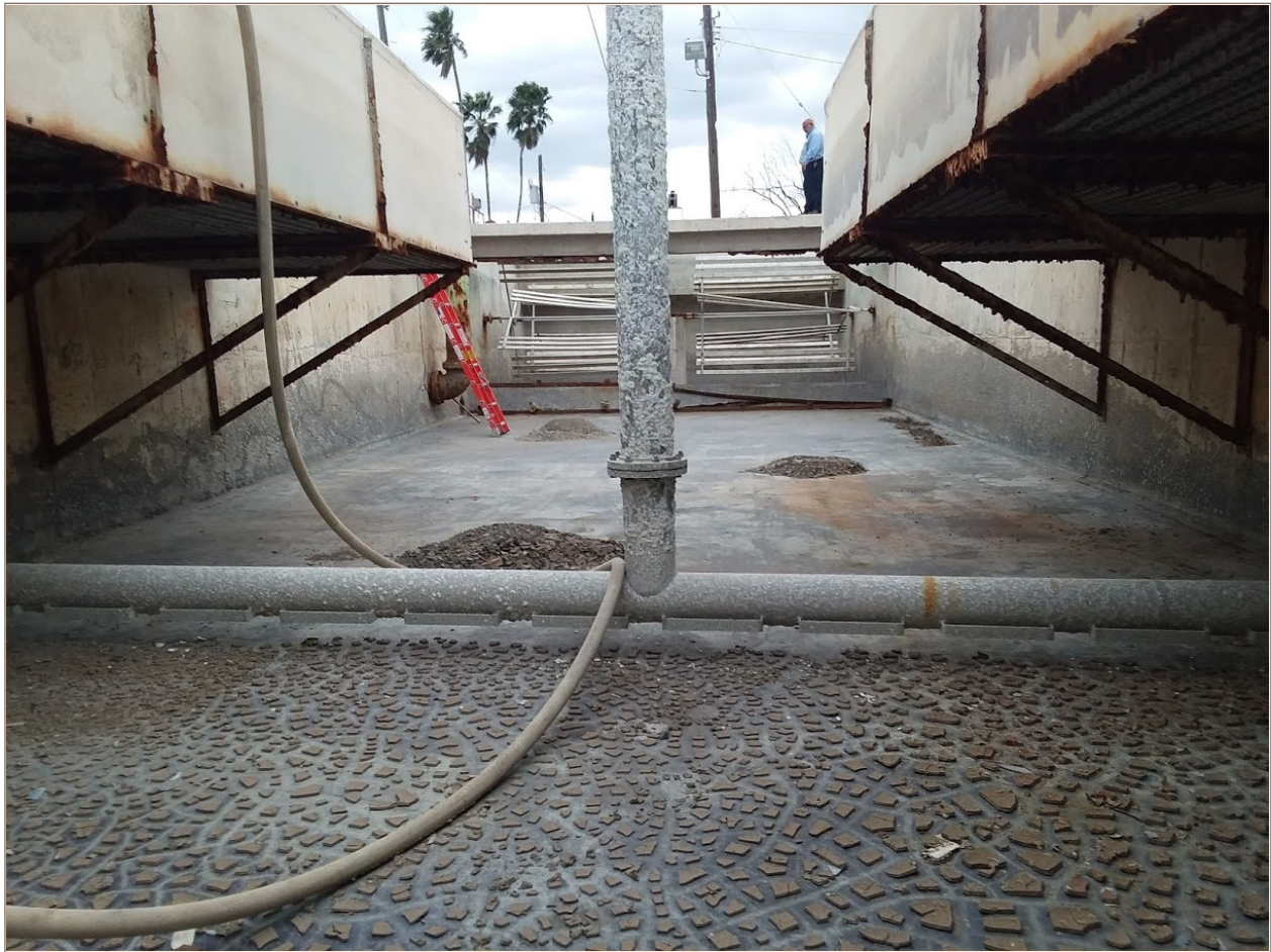
Existing Sludge Removal Equipment (Galvanized Pipe)
