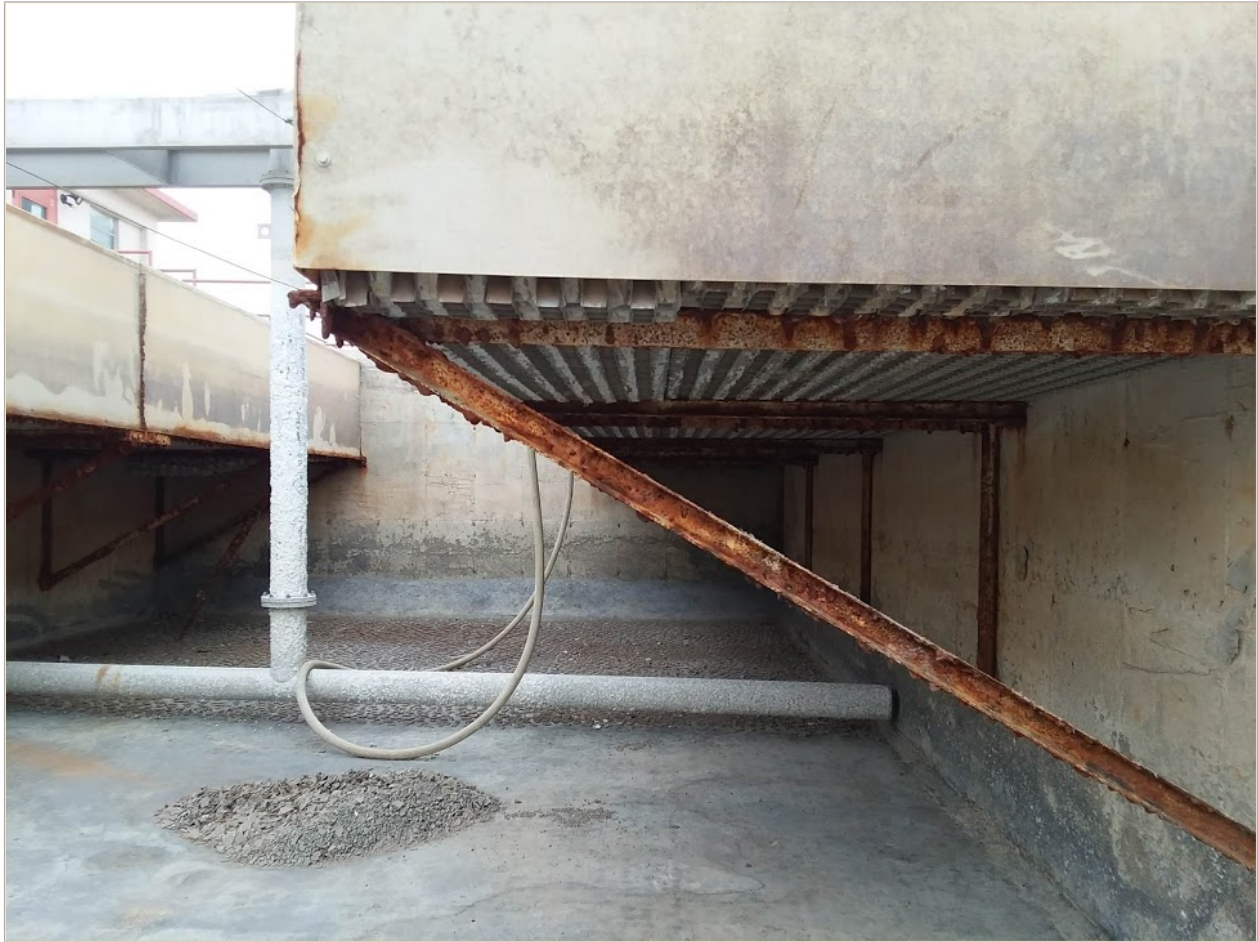
Existing North Tube Settler Module seen from bottom. The structural support members are in poor condition.
