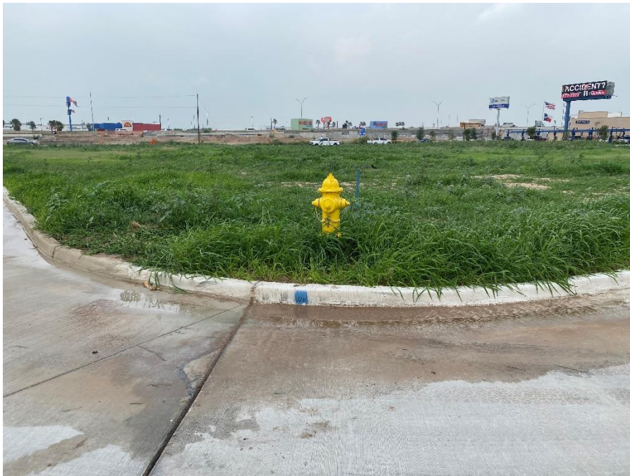
Curb must be painted red.
