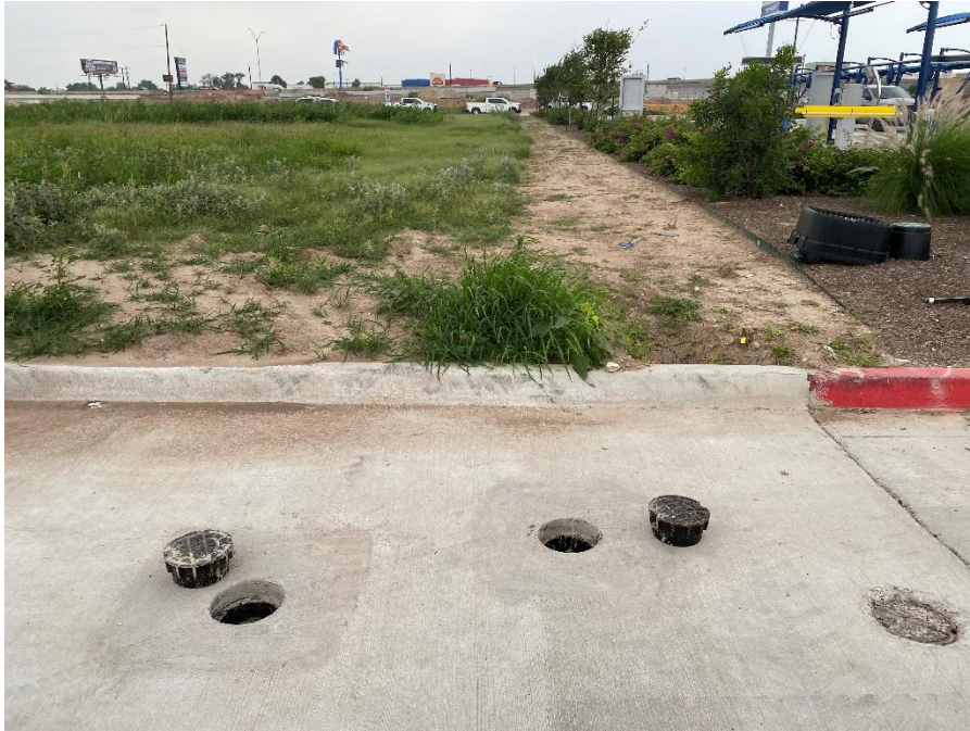
Water valves need to be included on the plans.
