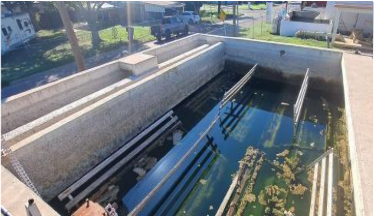
New rail tracks and wheels for sludge removal mechanism:
